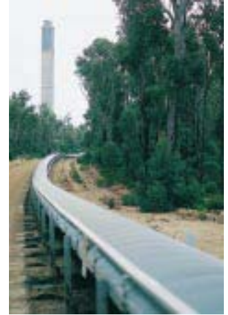
Above The conveyor belt delivering coal from Wesfarmers Coal's Premier mine to Western Power's new Collie power station, near Collie in Western Australia.
